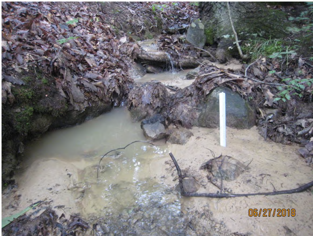
Photo 2: Sediment in stream ~685’ from LOD; Depth = 3”
