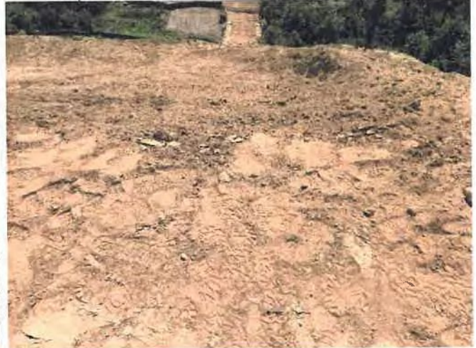
Fig. 4 Downslope from water bars with no storage depth
