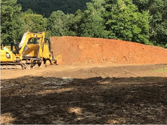
Fig. 3 Stockpile near AR G-I234, not protected / stabilized
