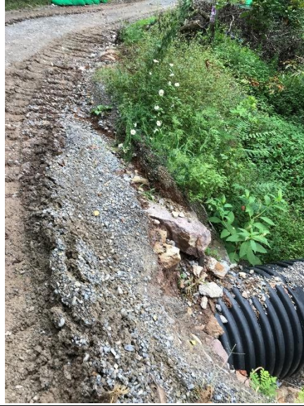
Fig. 4 Designated access road AR 241.01, observed erosion in curve
