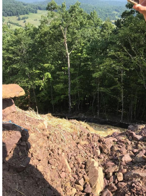
Fig. 2 Water bar with missing end treatment near station # 12024+00
