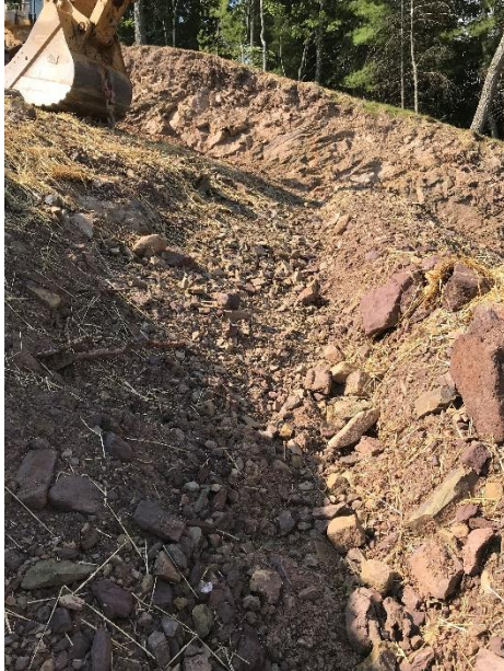
Fig. 1 Inadequate water bar near station #12024+00
