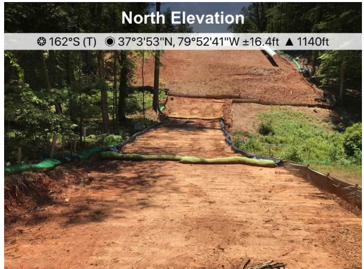
Fig. 4 ECD controls are in place at designated stream S-KL41
