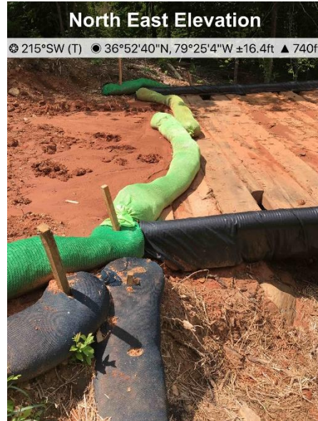
▪ Fig. 2 SB-8 remove accumulated sediment from bridge approach and repair undermined CFS
