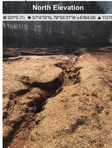
Fig. 4 St#13808+74 waterbar flow path has eroded and sump is filled with sediment
