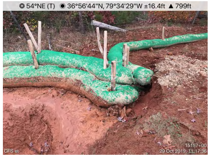
Fig. 10: STA 15157+00 – CFS end-treatment bypassed. Maintenance needed.
