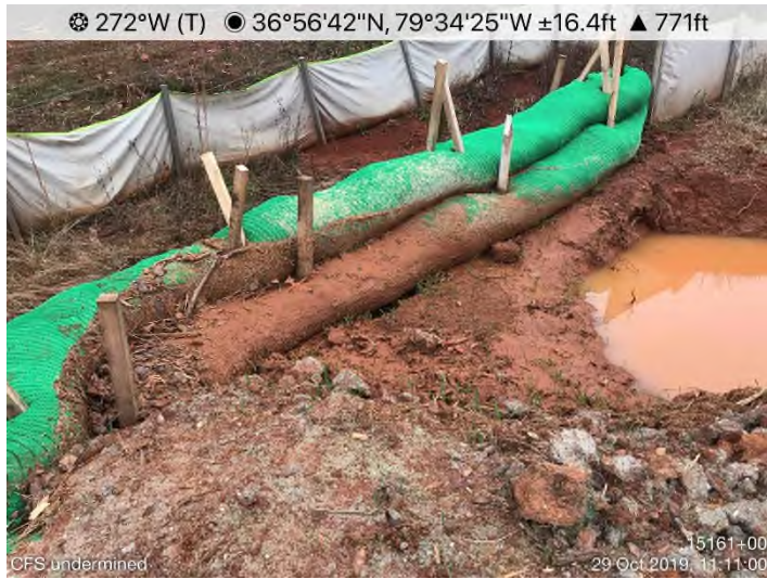
Fig. 9: STA 15161+00 – CFS undermined.
