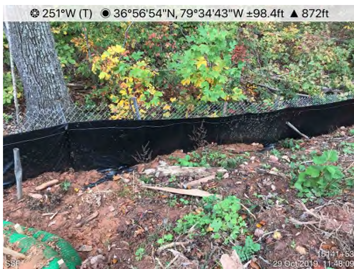
Fig. 11: STA 15142+00 – SSF undermined.
