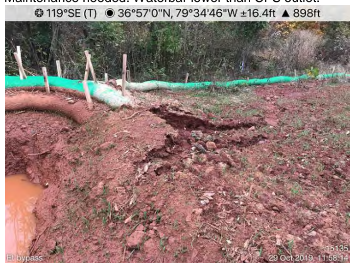
Fig. 12: STA 15135+00 – CFS end-treatment bypassed. Maintenance needed. Waterbar lower than CFS outlet.
