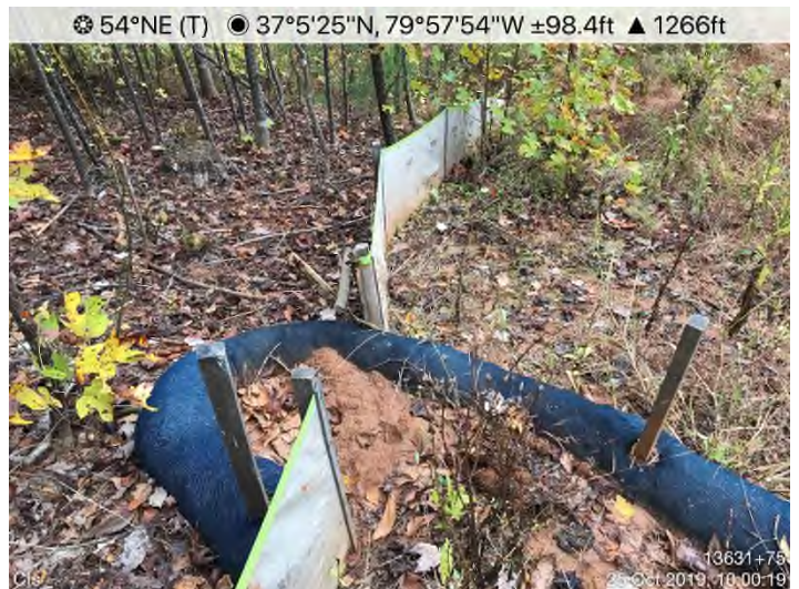
Fig. 4: STA 13631+75 – CFS maintenance needed.
