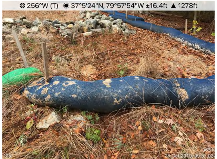
Fig. 2: STA 13631+00 – CFS undermined.
