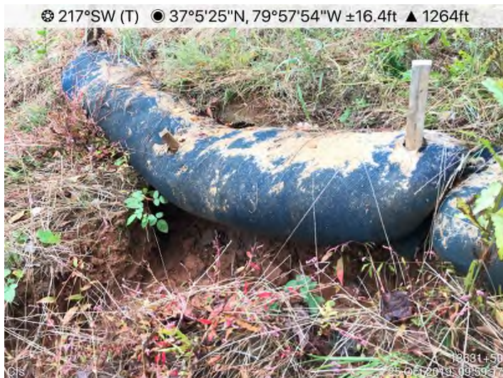
Fig. 3: STA 13631+50 – CFS undermined.
