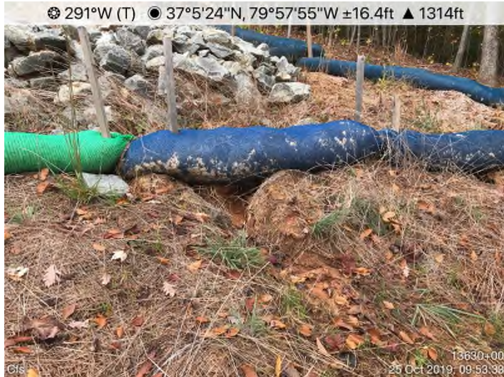
Fig. 1: STA 13630+00 – CFS undermined.
