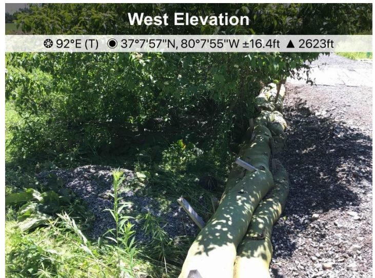
Fig. 2 Escaped road gravel off AR 288.
