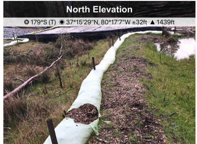
Figure 2: St12110+00 CFS requires maintenance.
