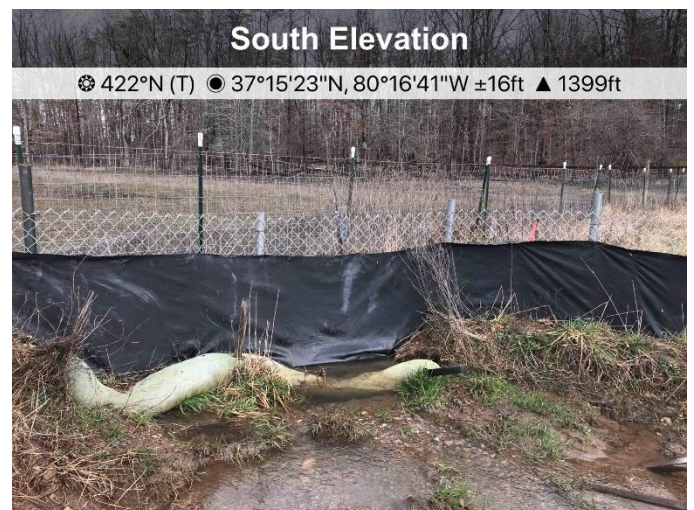
Figure 4: St17132+00 silt fence has been undermined and requires repair.
