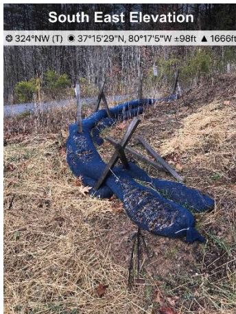
Figure 3: St1211+50 CFS triple stack requires maintenance
