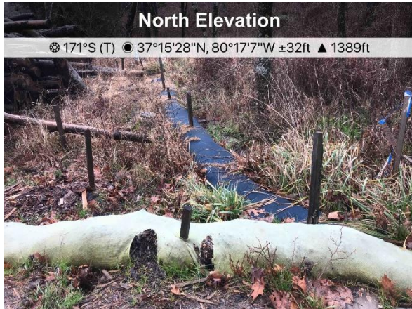
Figure 1: St12109+70 CFS requires maintenance.
