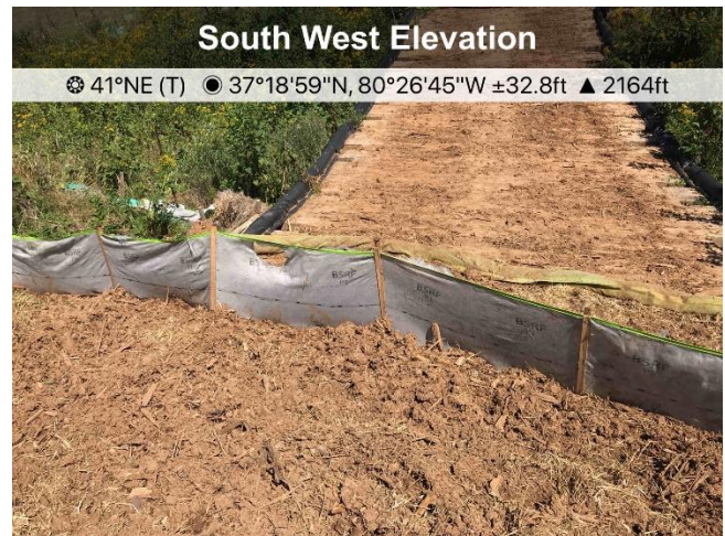
Fig. 4 MP216.4 P1 fence had a hole
