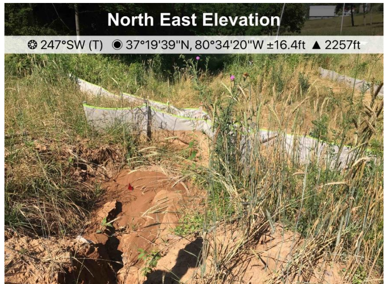
Fig. 4. St10964 sump requires maintenance
