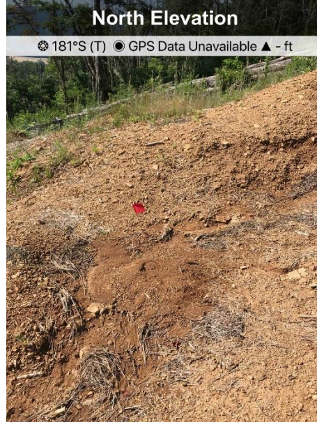
Fig. 2. St11014+00 waterbar flow path requires maintenance
