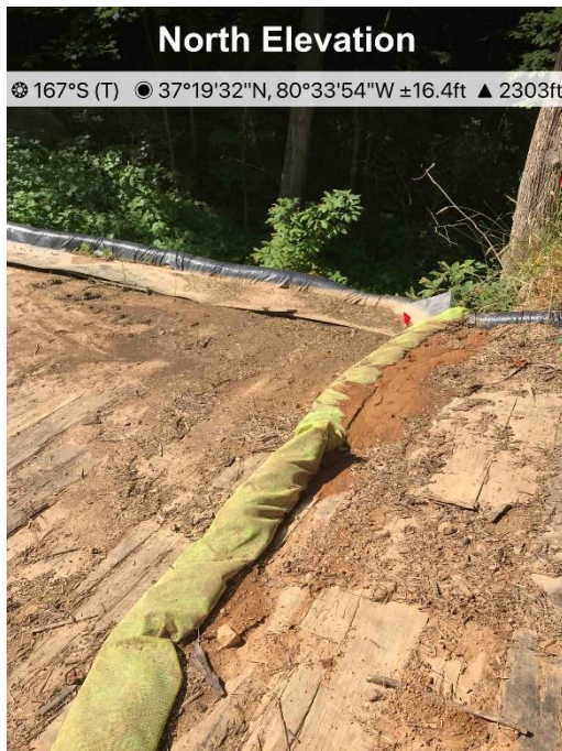
Fig. 3. MP207.9 waddle at bridge requires maintenance.
