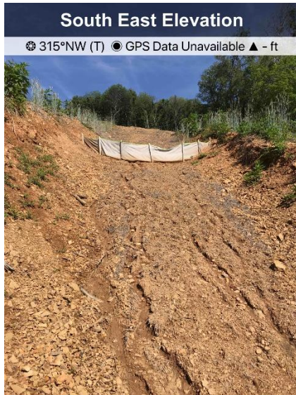
Fig. 1. St11014+00 rill erosion has occurred
