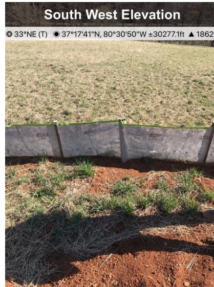
Fig. 2 St#11163+30 hole in P1 fence
