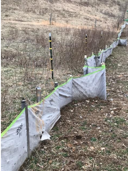
Fig. 1 St#11308+95 hole in P1 fence
