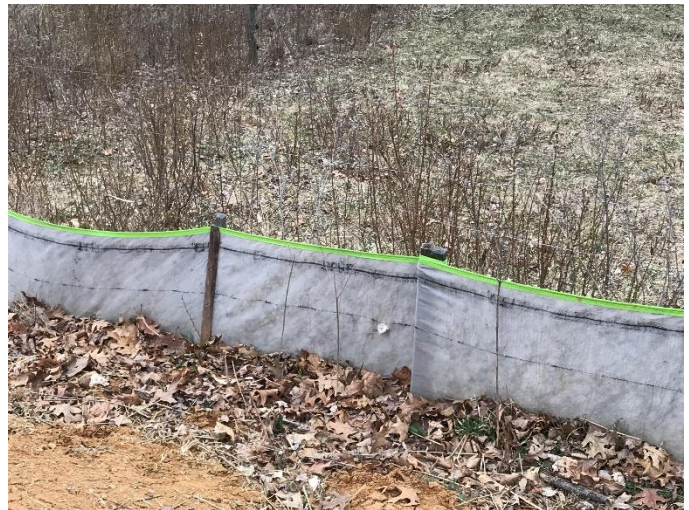
Fig. 4 St#11316+90 hole in P1 fence
