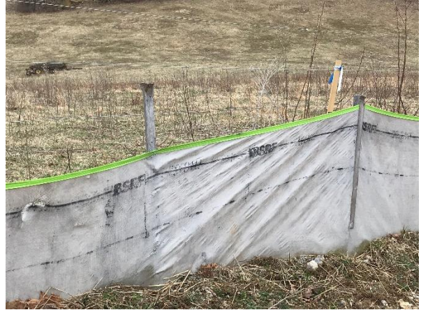
Fig. 2 St#11311+00 hole in P1 fence
