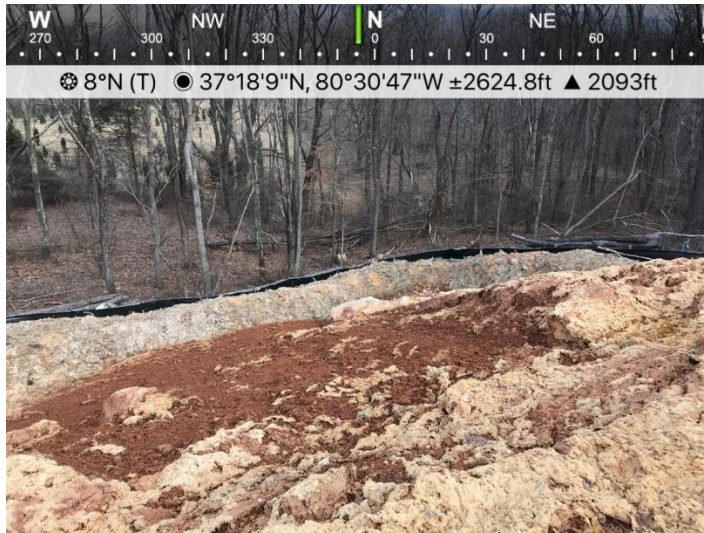
Fig. 3 At St#11529+50 slope has slipped and lacks stabilization.
