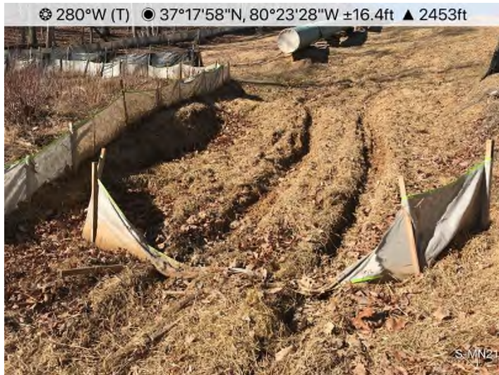
Fig. 1: STA 11687+00 – P1 maintenance needed.
