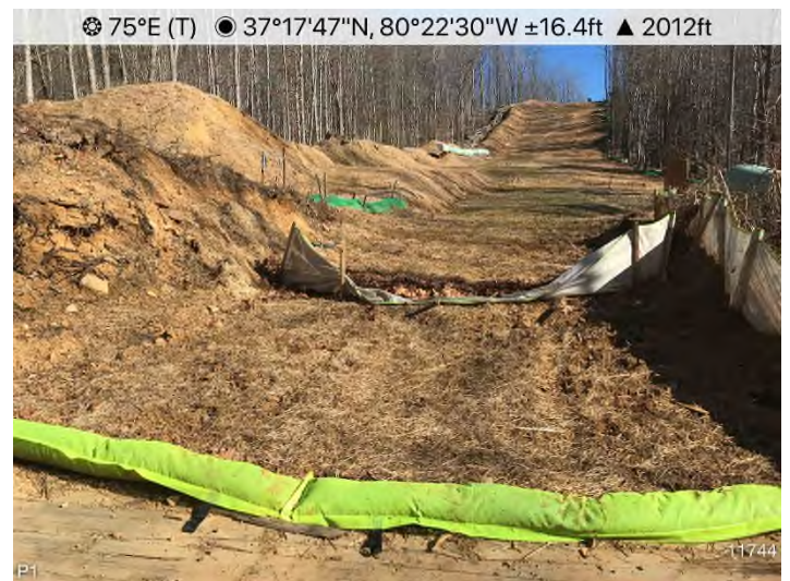
Fig. 4: STA 11744+00 – P1 maintenance needed.
