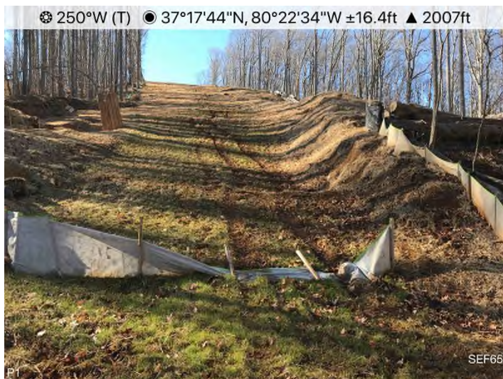
Fig. 3: STA 11740+00 – P1 maintenance needed.
