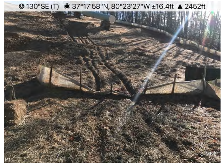
Fig. 2: STA 11687+00 – P1 maintenance needed.
