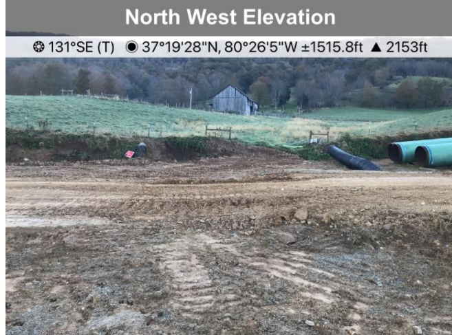
Fig. 1 At St# 11489 clean water diversion is inadequate.
