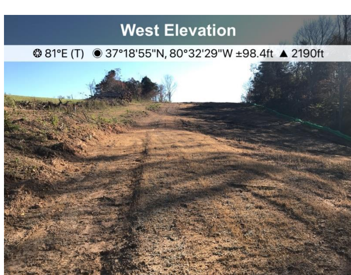
Fig. 3 St#11064+84-11073+00 is not adequately stabilized.
