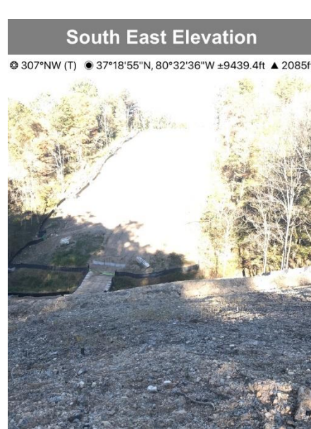
Fig. 2 St#11064+84-11073+00 is not adequately stabilized.
