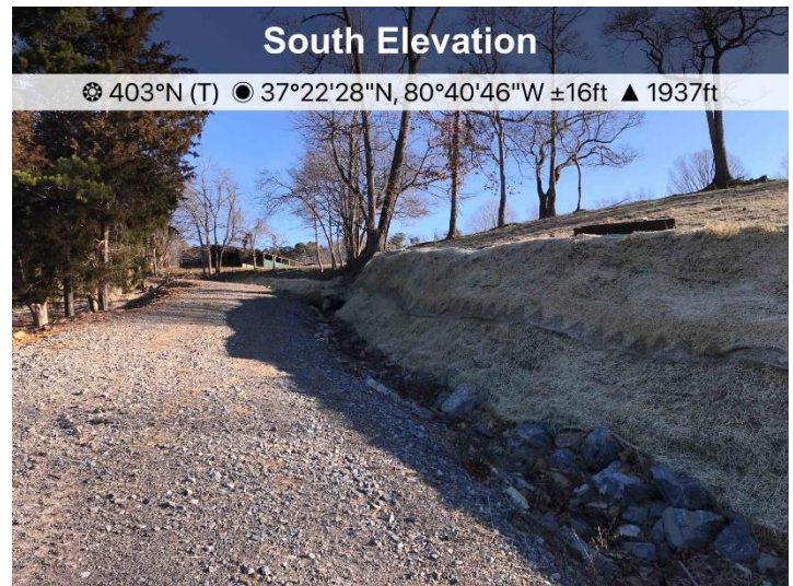
Fig. 4. At AR GI-234, additional matting has been installed.
