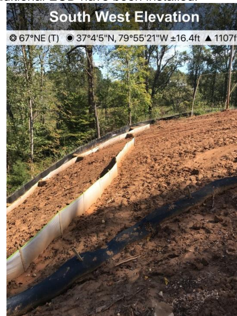
Fig. 4 At St#13819+00 MP261, slope has been repaired and additional ECD have been installed.
