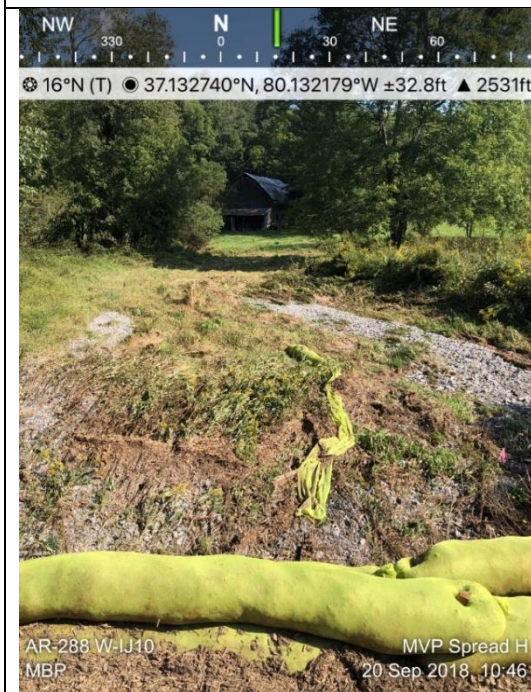
Description: Sediment off of AR-288
