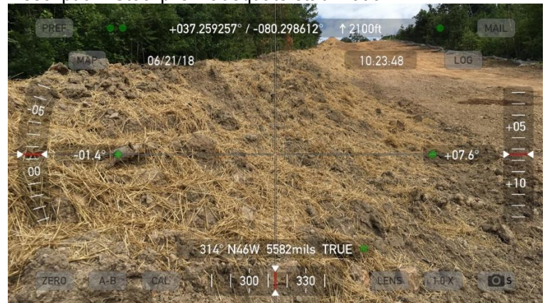
Fig. 4 Description: Stockpile inadequate stabilization
