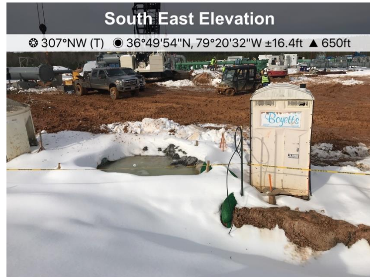
Fig. 2 Concrete washout at Transco station, noted for removal by MVP
