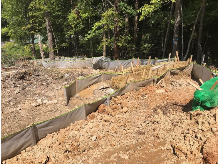
Area where E&S controls were overtopped and since repaired.
