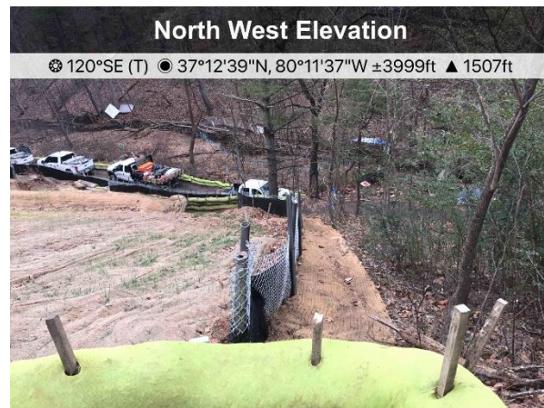
Figure 4: ECD's including sumps, and SSF are installed and appear to be functioning.
