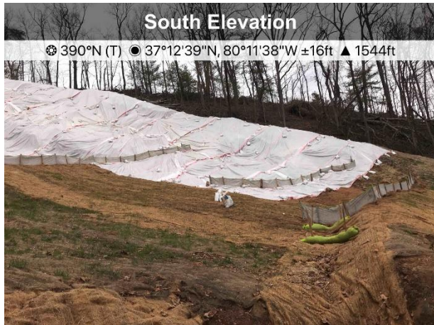
Figure 3: Near St12544+00 the stockpile slope has temporarily been stabilized with plastic sheeting, the remaining slope has been stabilized with blanket matting.
