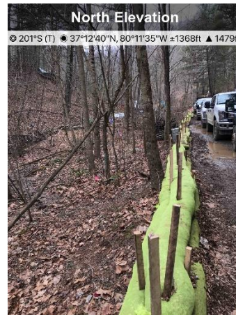
Figure 2: ECD's are installed and functioning along access road MN278.01, designated wetland W-EF5-PFO and designated stream S-EF20a.
