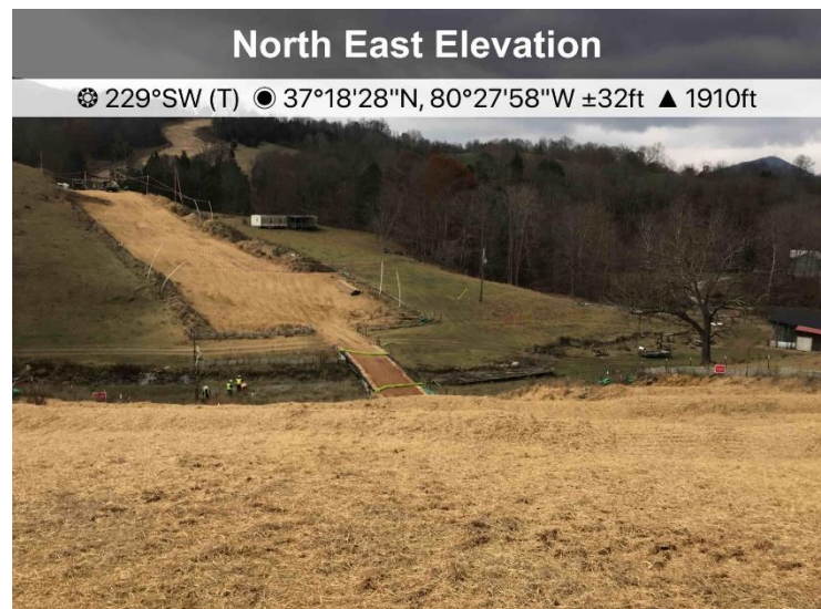
Fig. 4 Above designated stream S-KL43, ECD's in place and stabilization has been applied.
